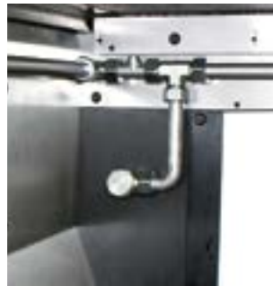
Flushing nozzles system
