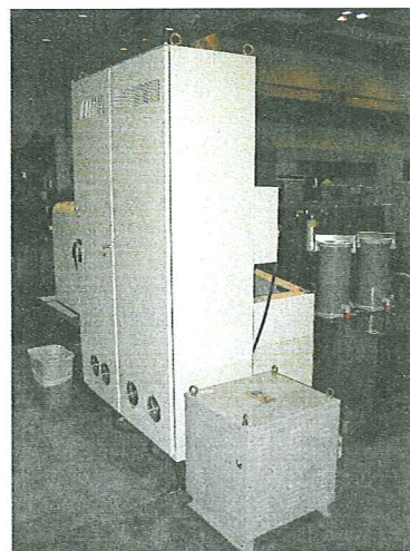
View of Electrical Cabinet
