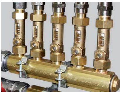
Five separate cooling circuits
