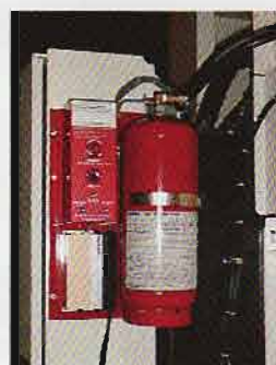
Automatic fire extinguisher (Note)
